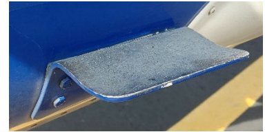
(Above: A fuel step on a C-182) Watch it flex when someone stands on it. Eventually, it will rip the metal behind it which is a specialized repair job done up at a shop in New Jersey.
